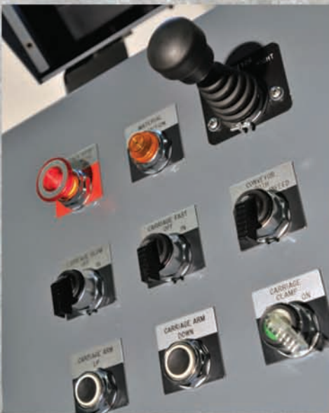
Typical control pedestal
